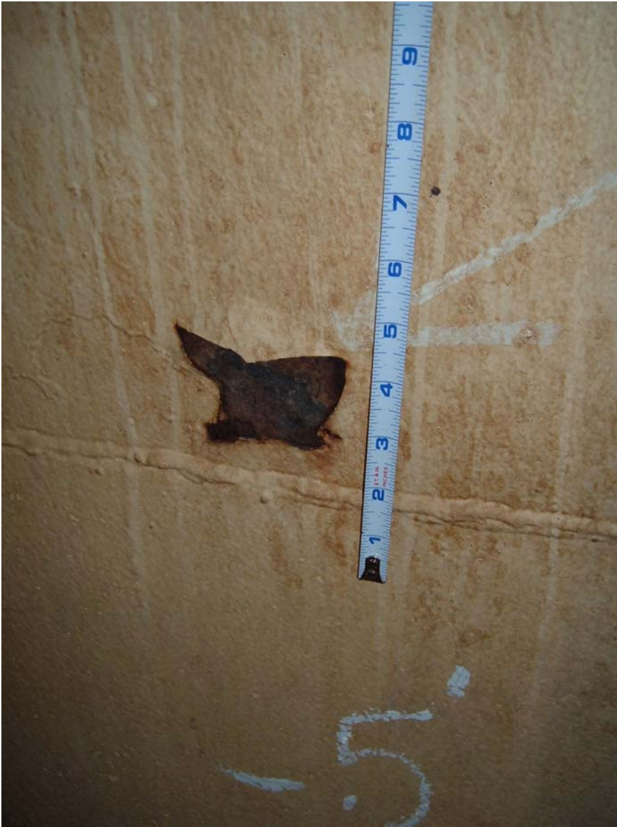
Fig. 15 – Isolated major corrosion on east side of lower second shell course
