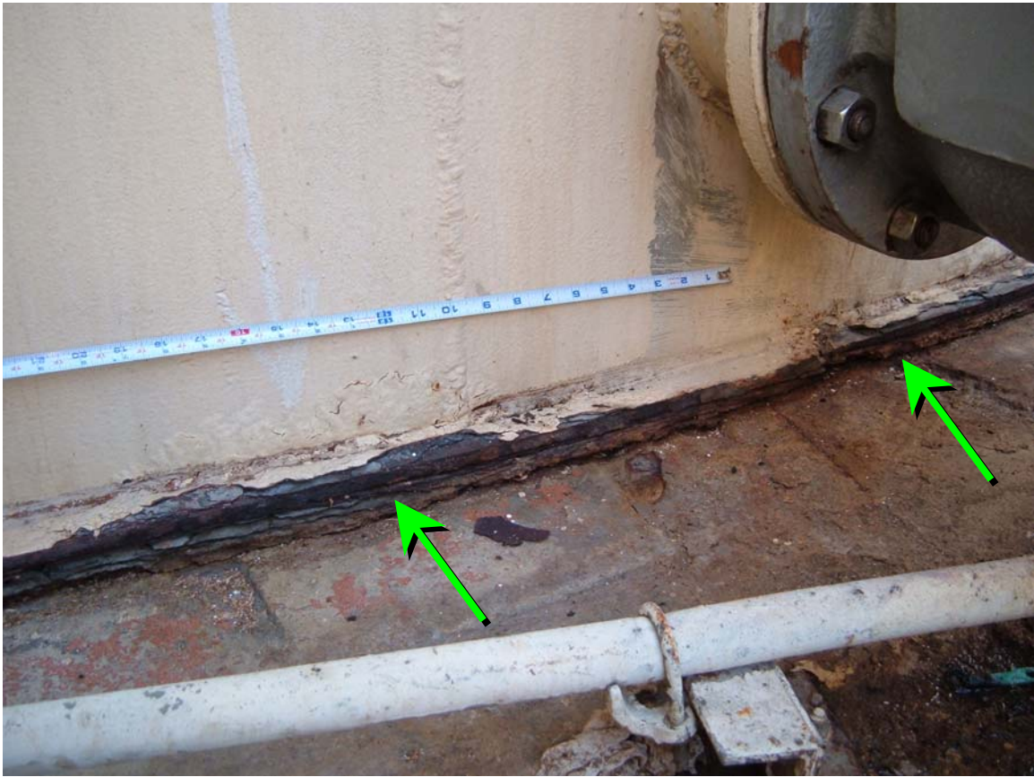
Fig. 1 – Major scale corrosion of floor protrusion
