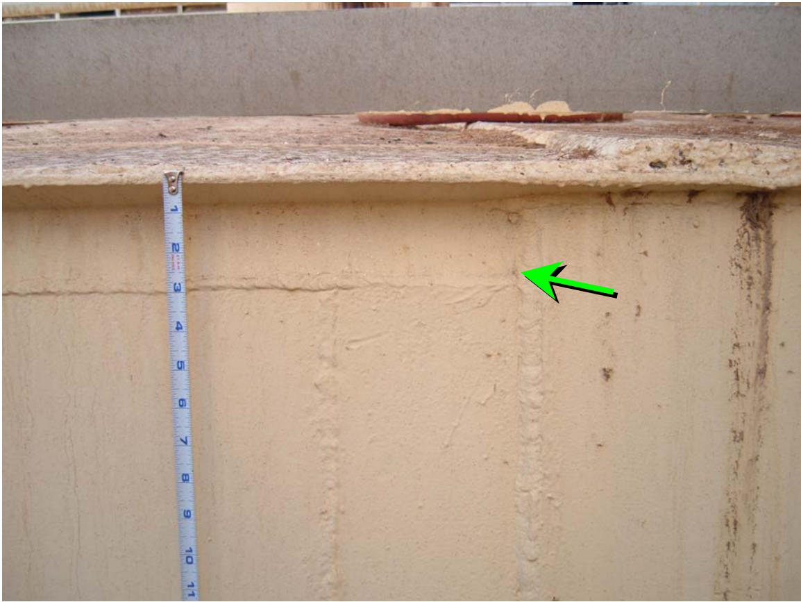
Fig. 7 – Shell plate misalignment near roof on the south side
