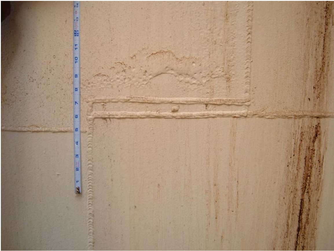
Fig. 5 – Weld spacing does not meet API-650 or good engineering practices
