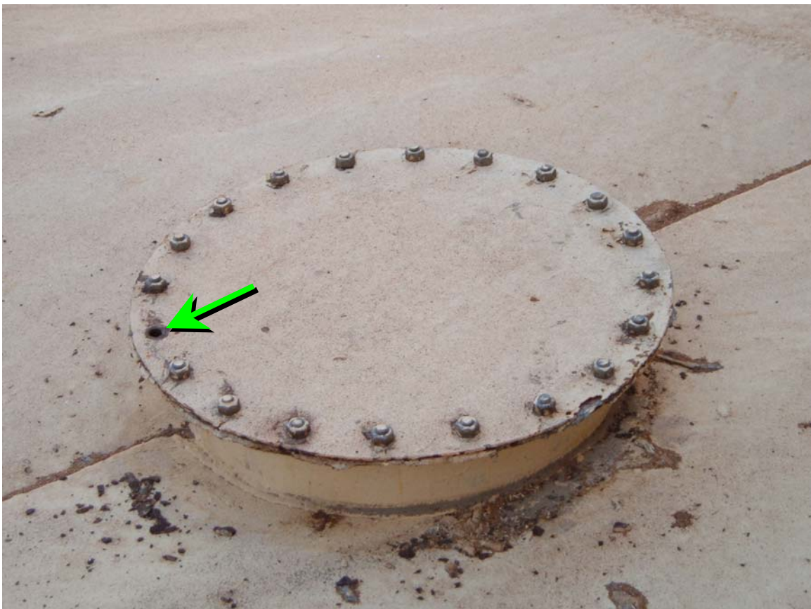
Fig. 8 – Roof manway is corroded and missing one bolt
