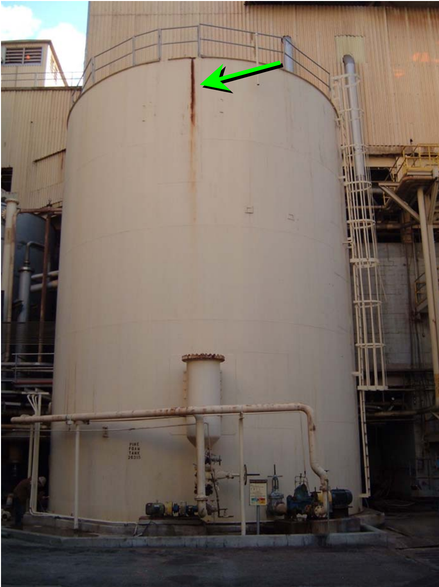
Fig. 9 – Corrosion on west side and multiple shell insert plates with non-rounded corners
