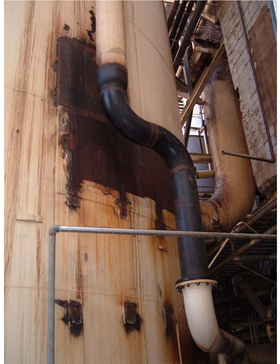
Fig. 12 – Multiple attachments with non-rounded corners, poor weld quality, and major corrosion (south-east side)
