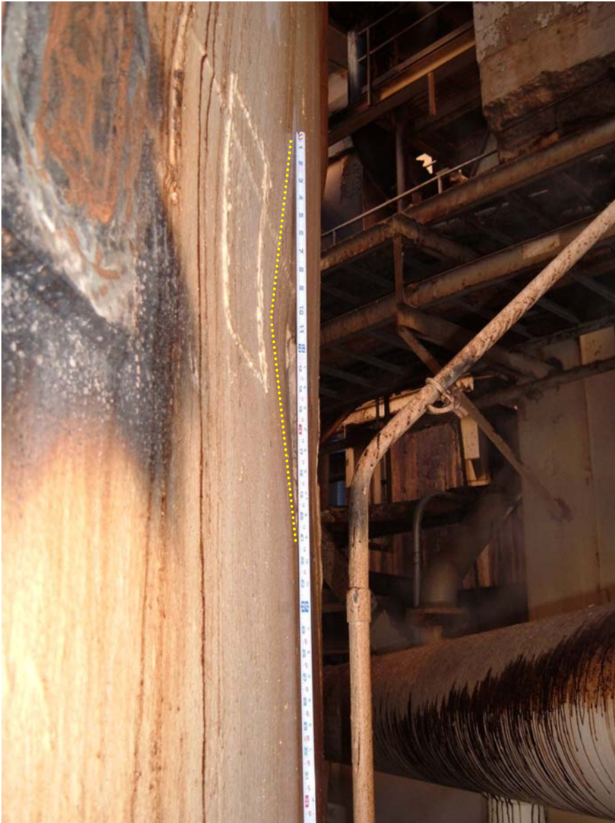
Fig. 13 – Minor shell deflection on upper second shell course (south-east side of tank)
