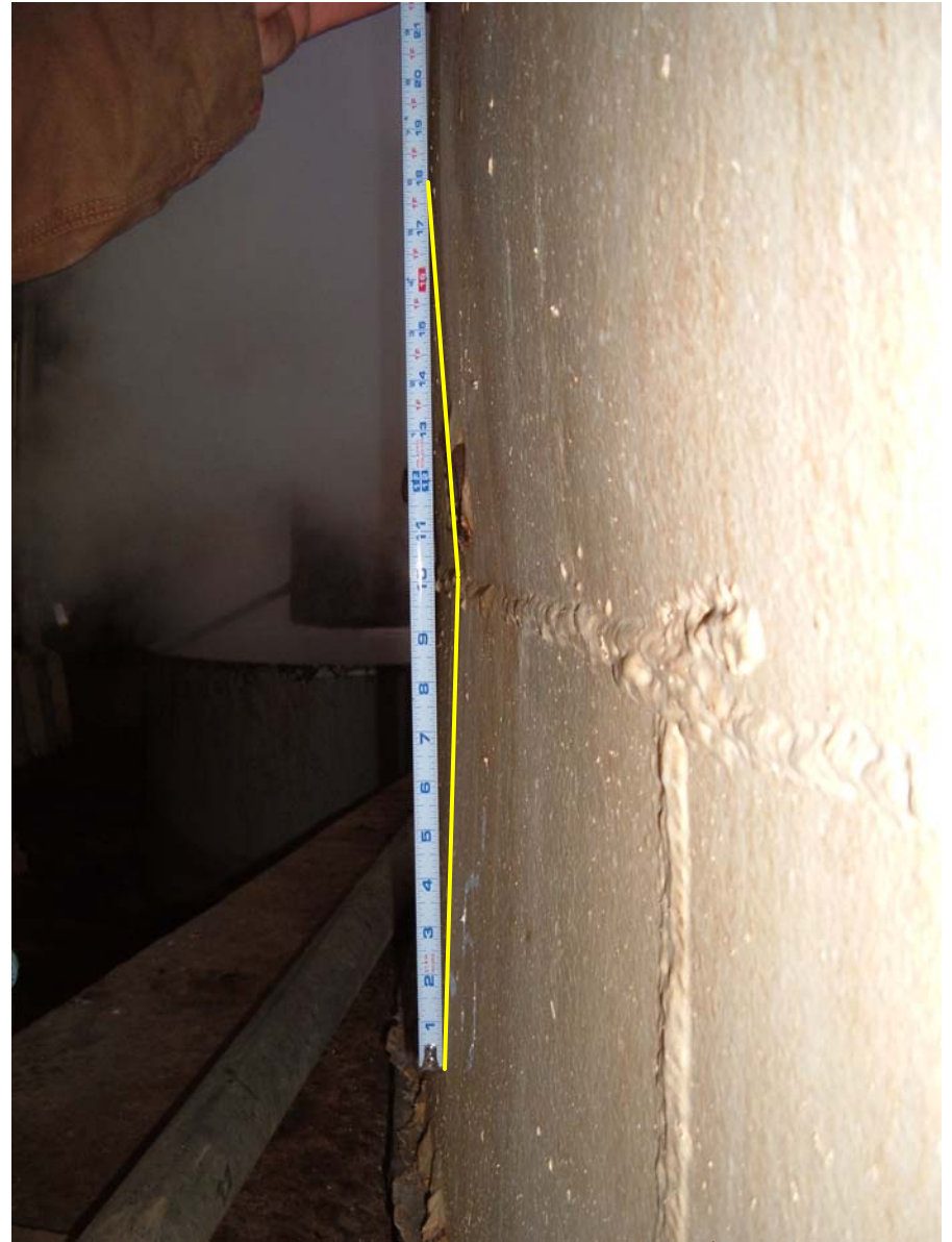
Fig. 16 – Minor shell deflection between 1 st and 2 nd shell course on east side of tank
