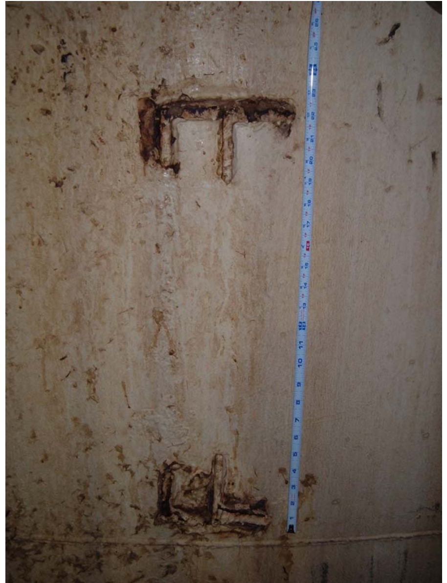
Fig. 14 – Attachments on lower second shell course on the east side of tank
