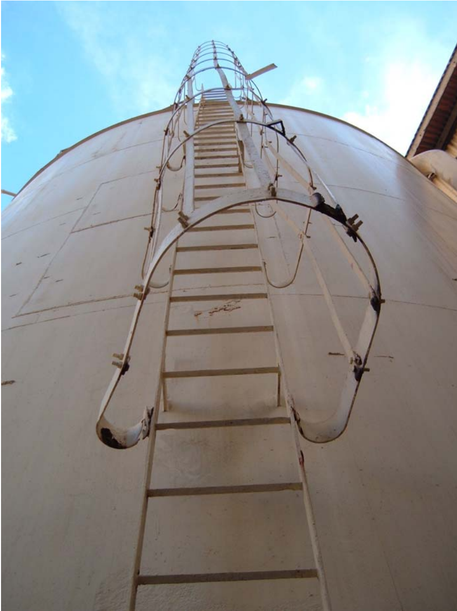
Fig. 11 – Major scale corrosion on ladder. Lower rungs have been removed to prevent access
