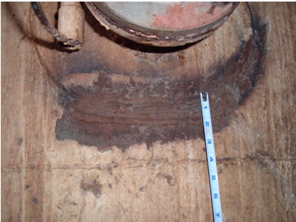
Fig. 4 – Poor and excessive weld on penetration reinforcing plate (East side)
